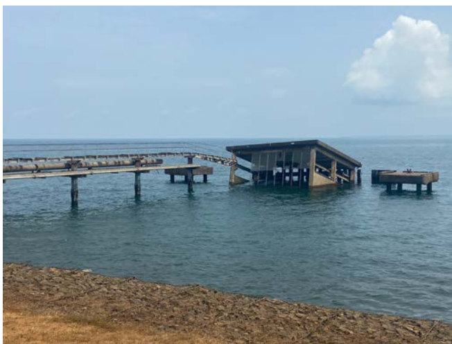
(b) Broken pier
