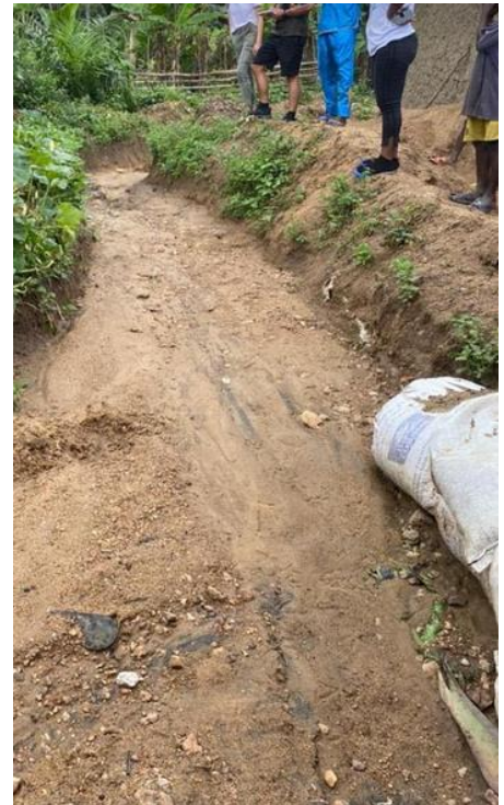
Figure 3 – A larger 40inch drain into junction, with banks, slopes and reinforced with sandbags protecting houses. Foindu Mameima
